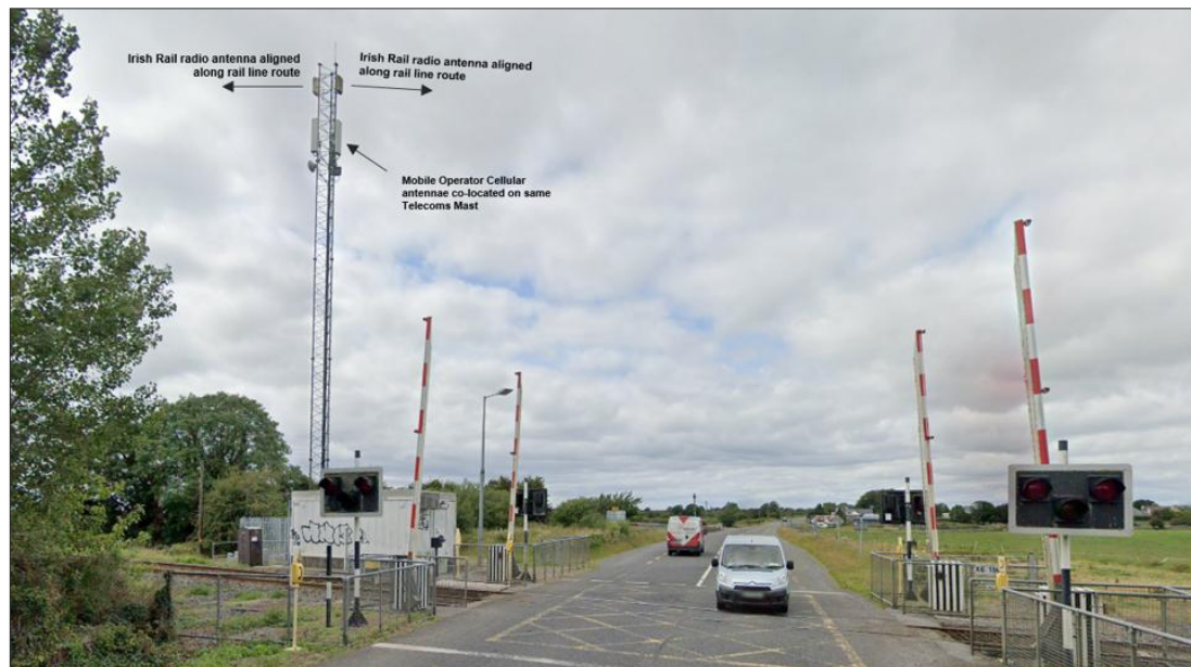
Figure 13. Example of GSM-R Train Radio installation using Directional Sector Antennas
